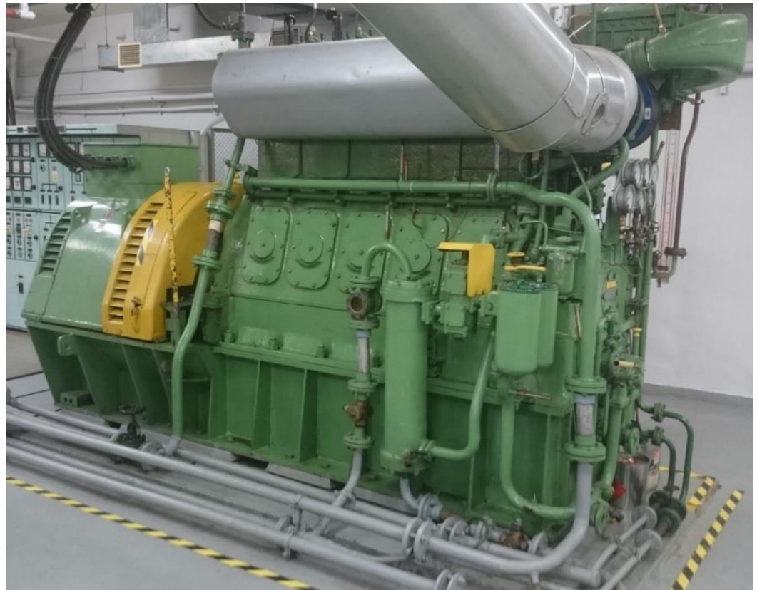
Figure 1. Sulzer 5 BAH 22 engine and associated circulating lubrication system.
